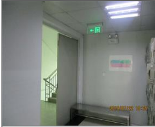
Photo of fire safety equipment Emergency exit of workshop.JPG
