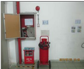
Photo of fire safety equipment Fire facilities at production building.JPG
